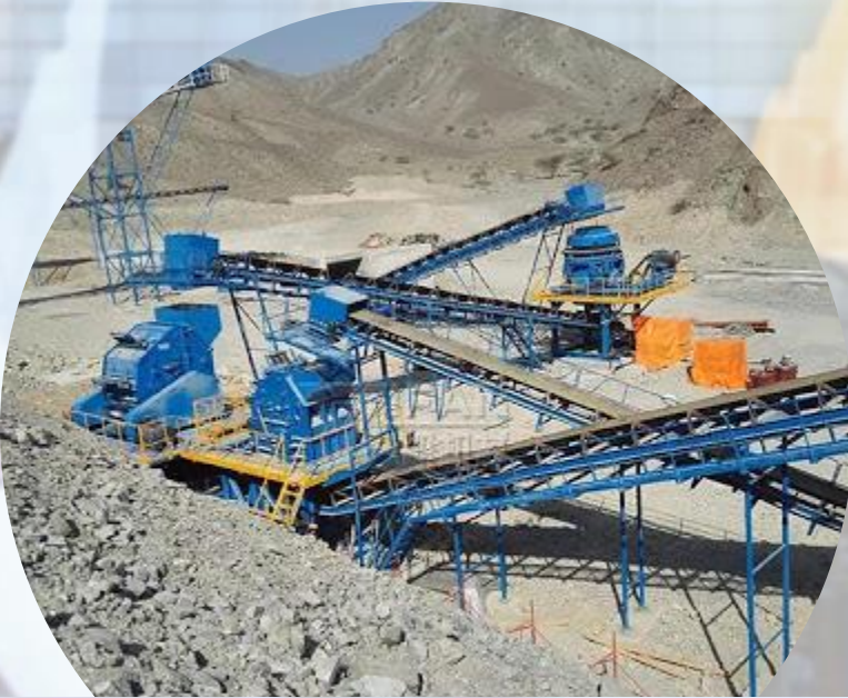
Mining Ore crushing plant
